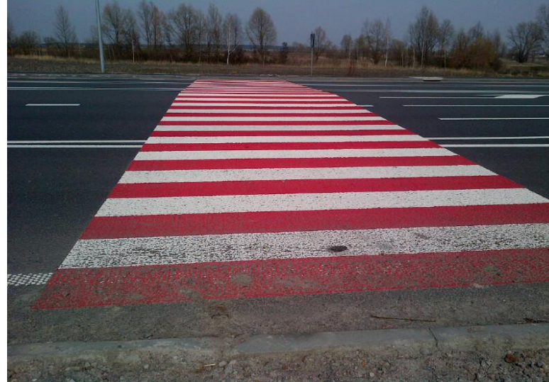
Unsafe pedestrian facilities
