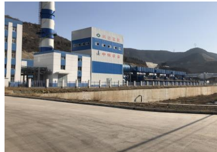
VAM destruction plant with 25 MW steam turbine to generate electricity Working Mine, Yangquan, Shanxi, China
