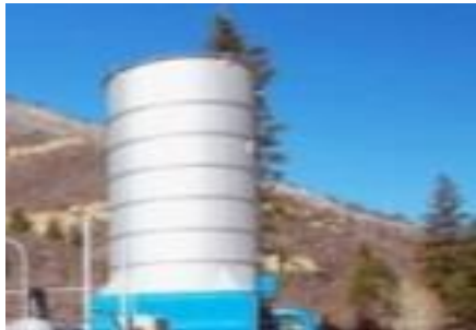
Abandoned Mine Methane Flare Colorado, USA
