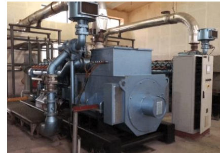
Gas-fired Generator - Working Mine, Pingdingshan, China
