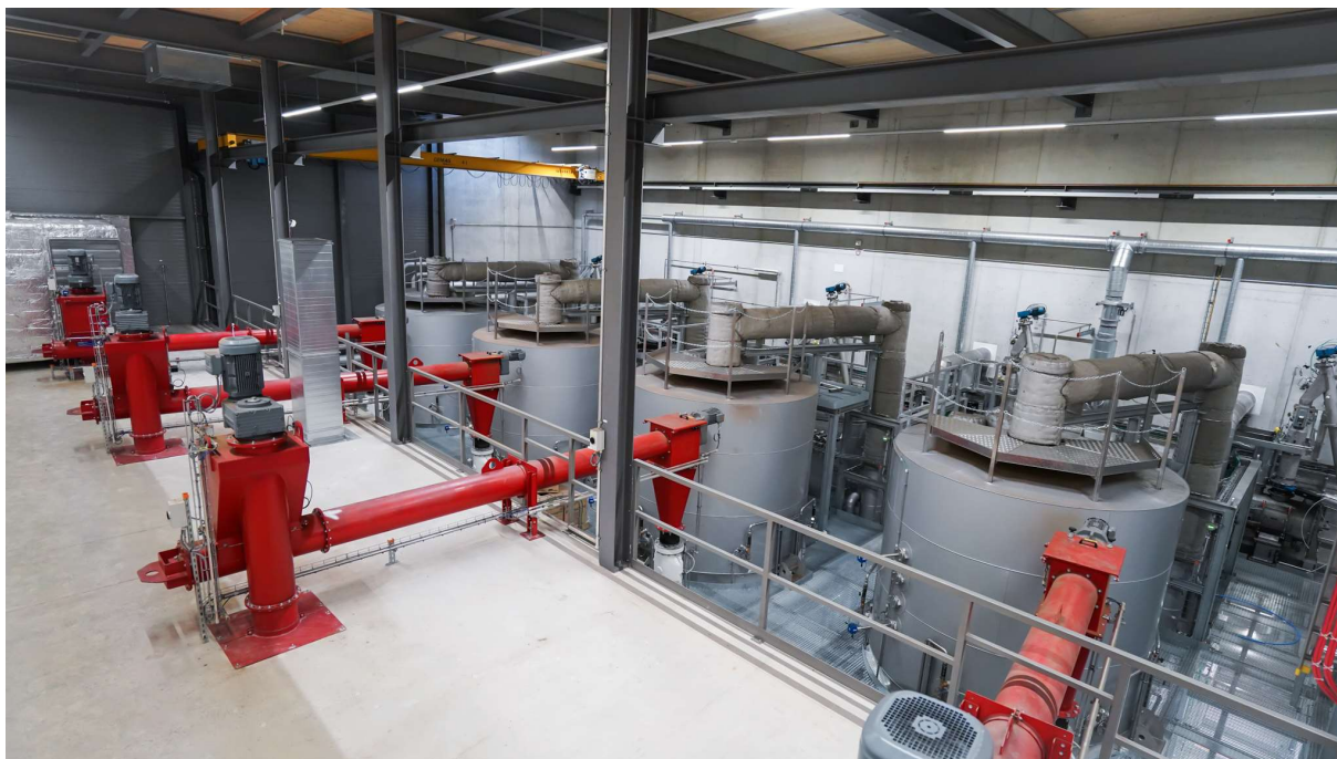
Fig. 38 The four floating fixed-bed reactors at the wood-fired CHP plant in Frauenfeld
