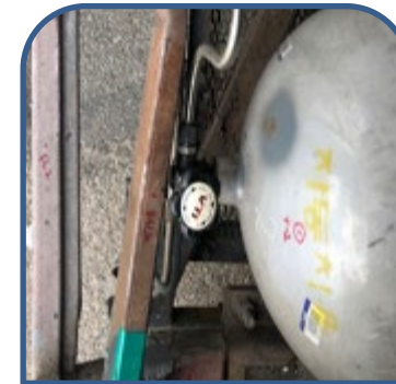
<Fracture of fuel valve>
