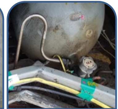
<Disconnected fuel line>
