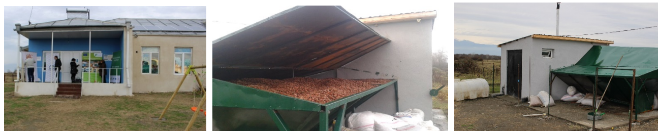
Picture 6: Solid Fuel Stove, Boiler House with Hazelnut Shell Reservoir – Erismedi Kindergarten
