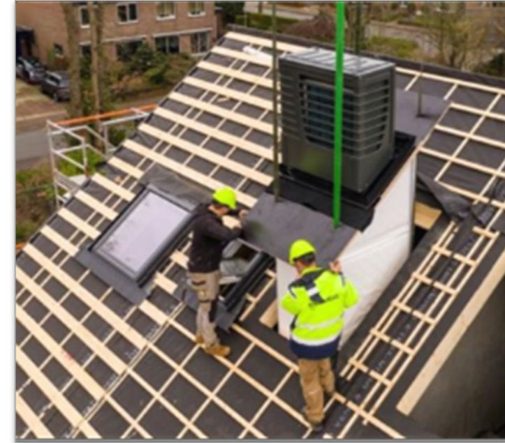
Prefab energy modules
