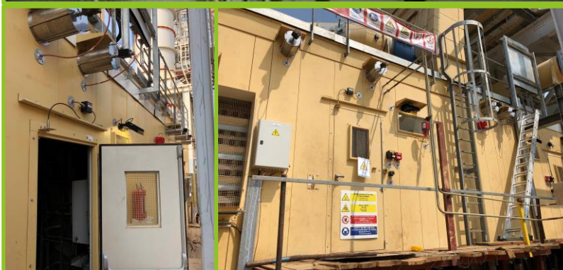
Gas Turbine Generator Frame 5
