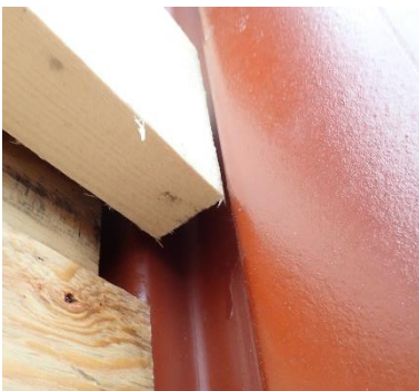
Figure 1 Beam too short
