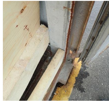
Figure 24 Beams too short
