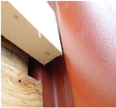
Figure 23 Beam too short
