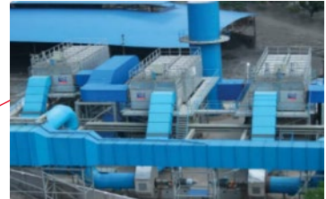
Datong mine, 2011 370,000 Nm 3 /h Hot water generation
