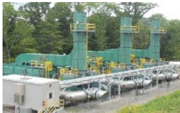
Verdeo McElroy mine 2012 250,000 Nm 3 /h 6 MW steam turbine
