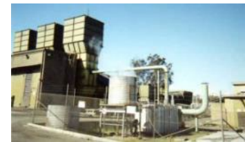
Appin Colliery mine, 2001 10,000 Nm 3 /h
