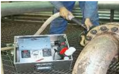
Oil & Gas Systems
