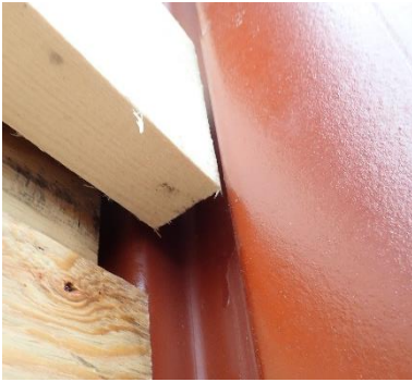
Figure 1 Beam too short
