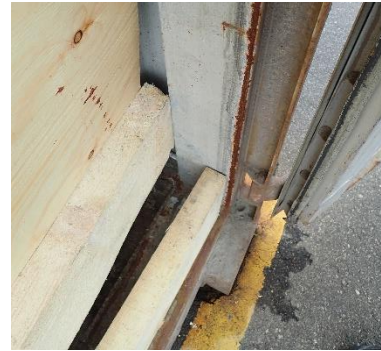
Figure 2 Beams too short
