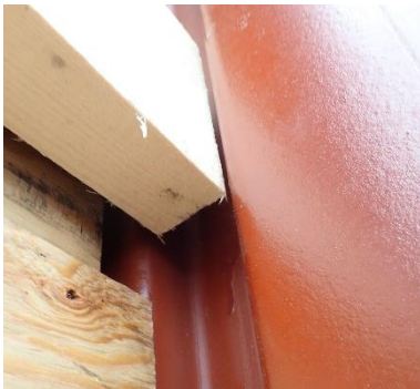
Figure 23 Beam too short
