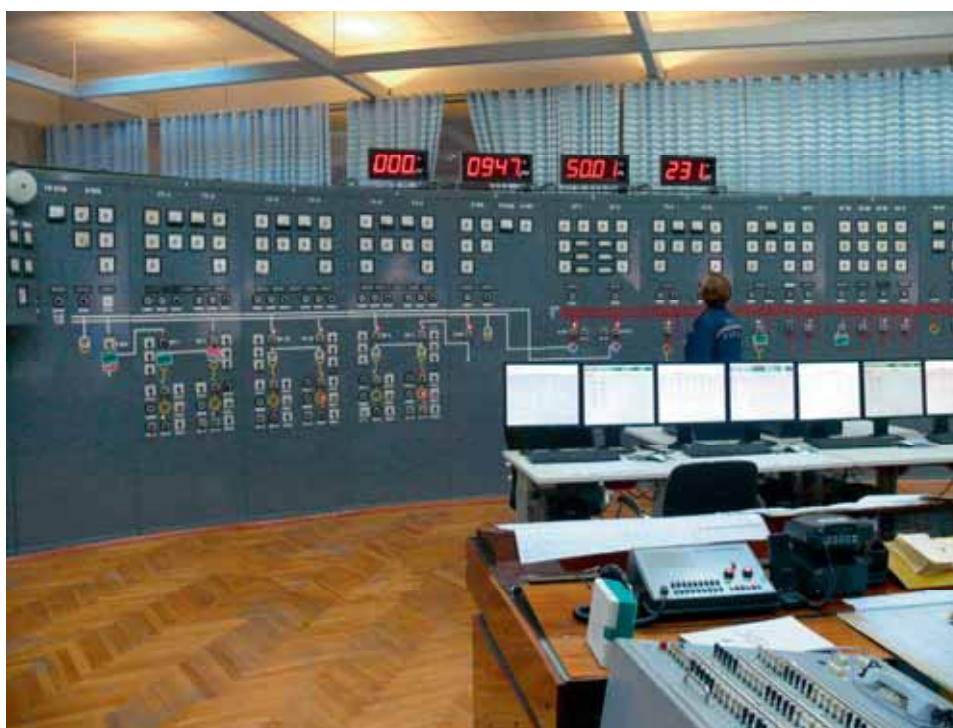
Photo 11.1: Nurek HPP control center
