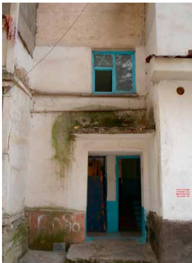
Photo 13.2: Poorly maintained multi-apartment housing stock, Dushanbe
