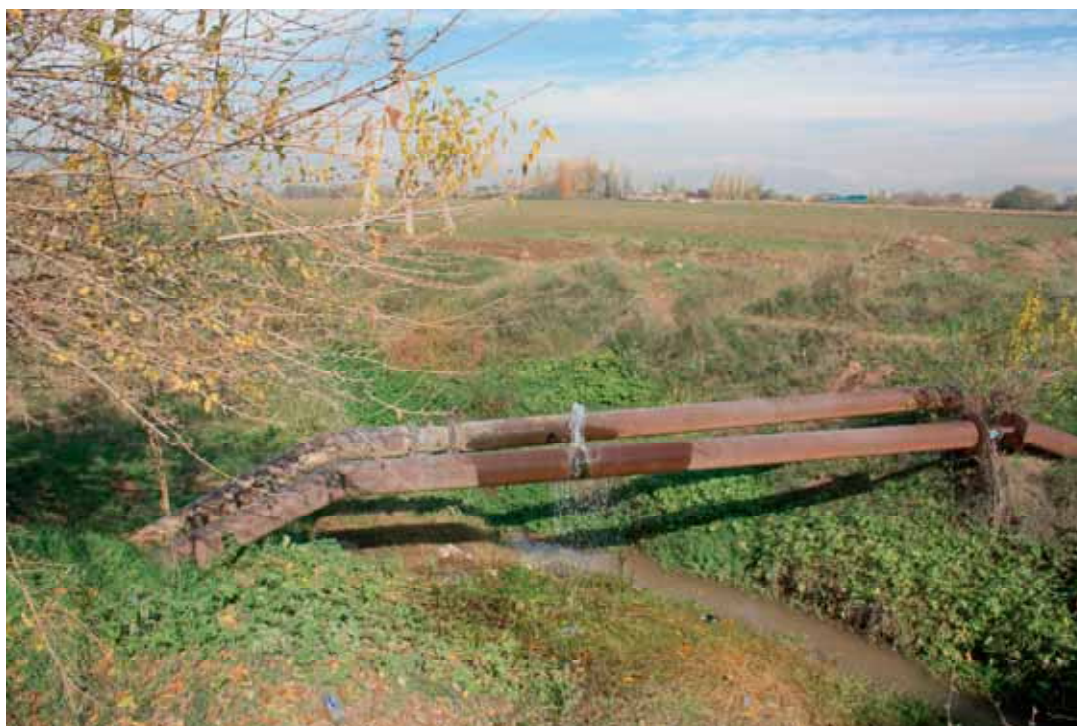
Photo 3: Breakdowns in irrigation water pipes
