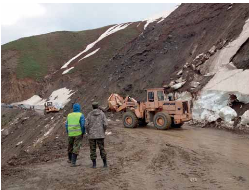
Photo 12.2: Landslide on Dushanbe-Khujand road
