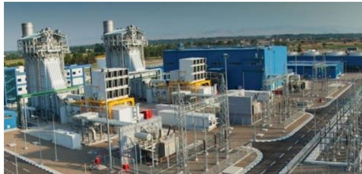
Gardabani Power Plant 1 and 2
