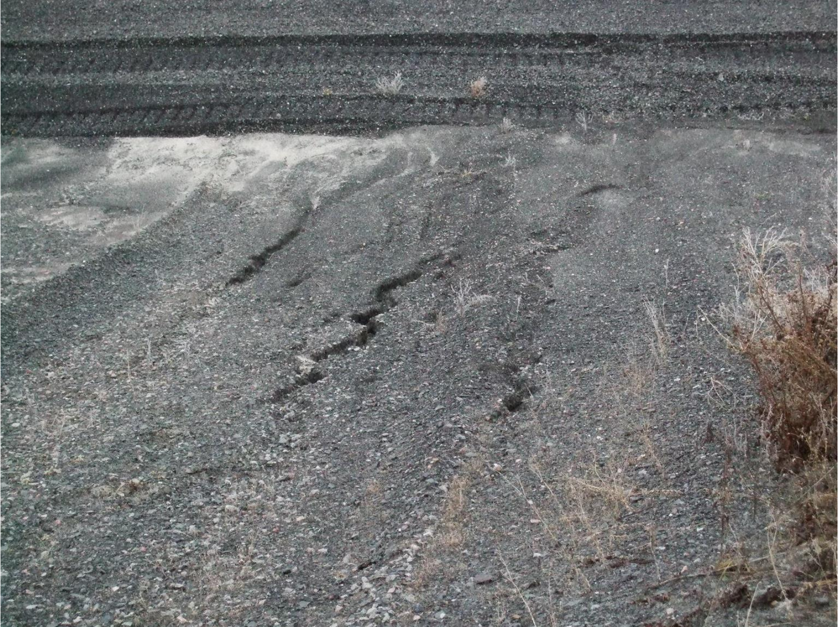
External slope of the tailings dam: rain washouts. In these places, gullies may occur
