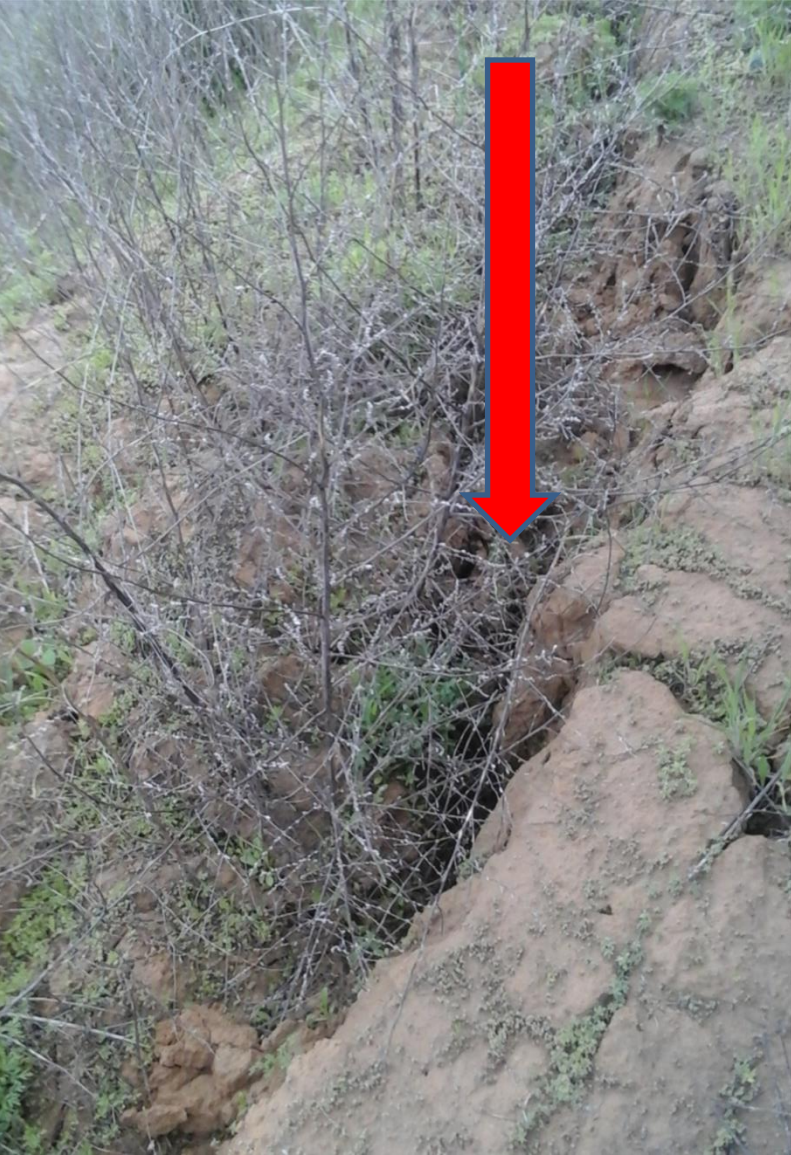
The outer side of the tailings dam. Landslide Breakaway Crack
