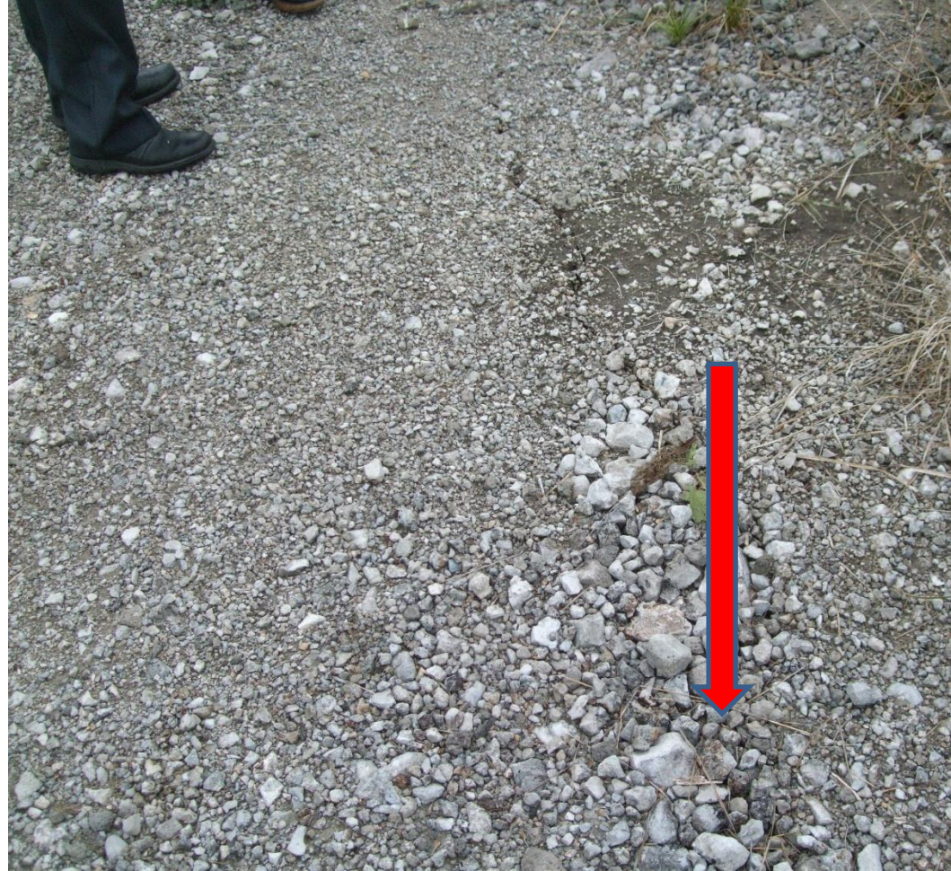
The crest of the tailings dam. The breakaway crack is an implicit sign of an incipient landslide
