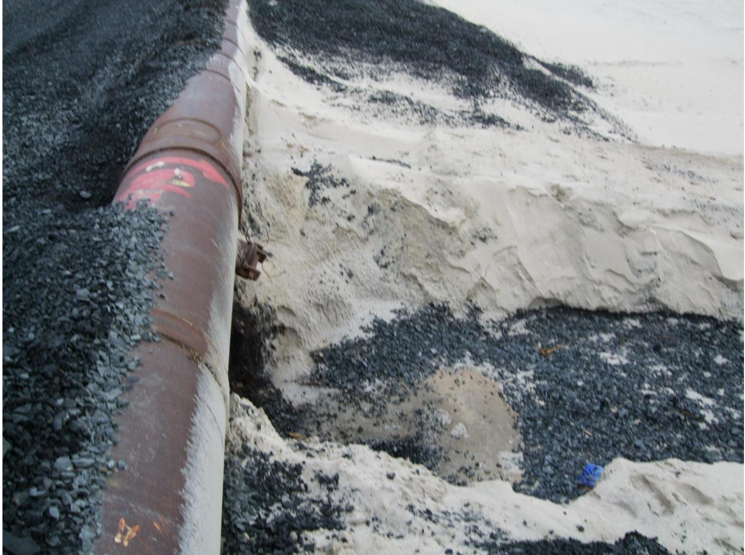
Internal slope of the tailings dam. Erosion due to sludge pipe leaks
