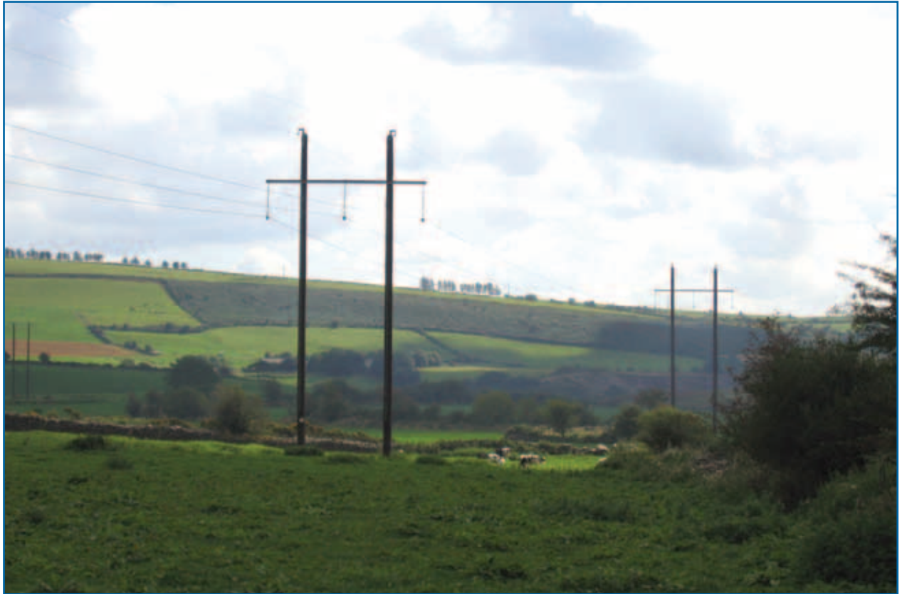
Figure 8.3: An existing 110 kV single circuit line
