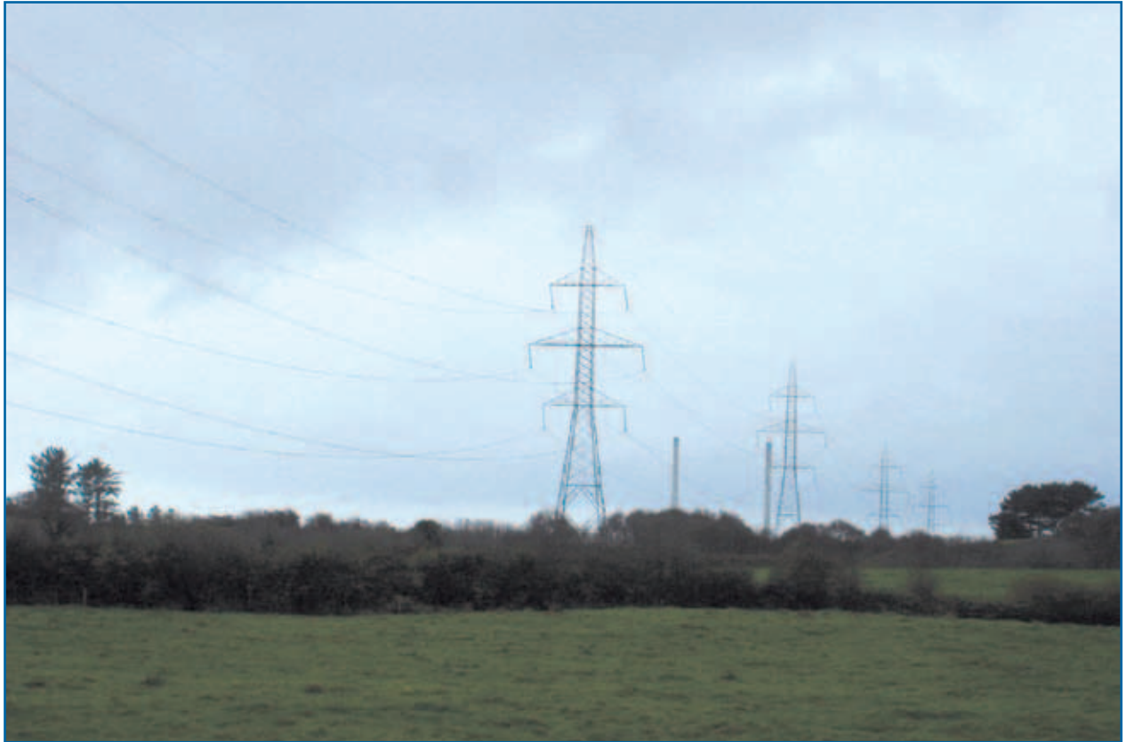
Figure 8.2: An existing 400 kV double circuit line close to Moneypoint generating station in County Clare
