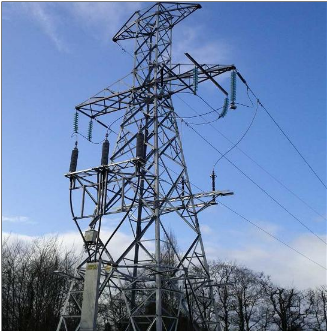
Figure 8.4: Photograph of a 110 kV Earthwire Line/Cable Interface Mast
