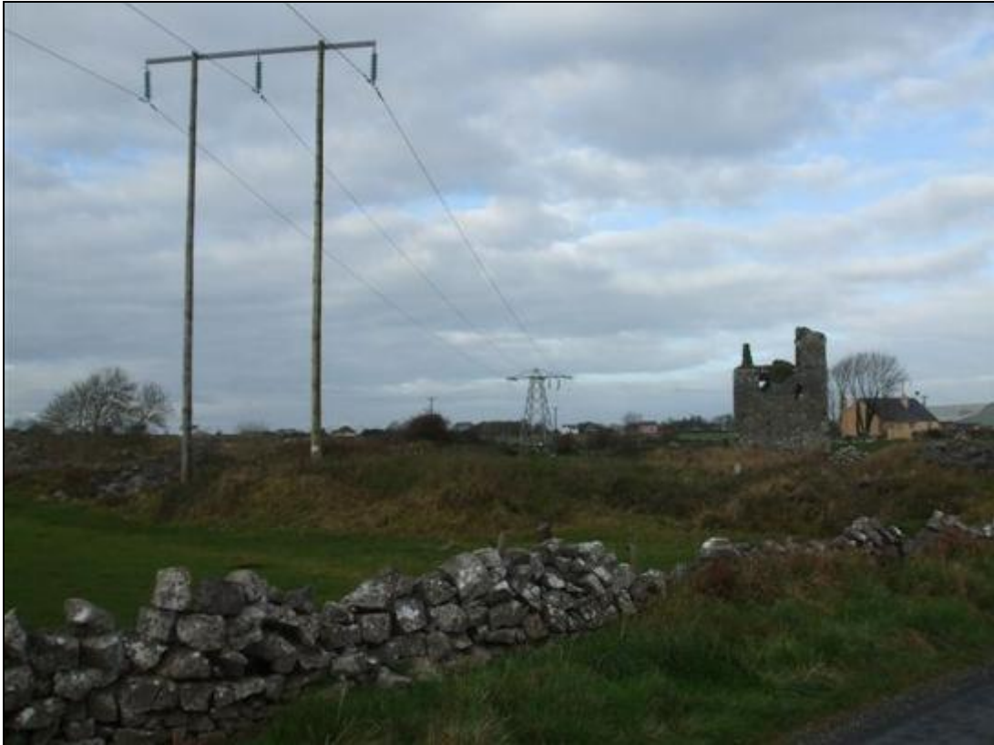
Figure 8.10: Photograph of a 110 kV Non-Earthwire Poleset
