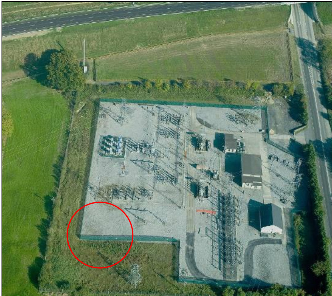
Figure 8.11: Photograph of the Existing Kilkenny Substation
