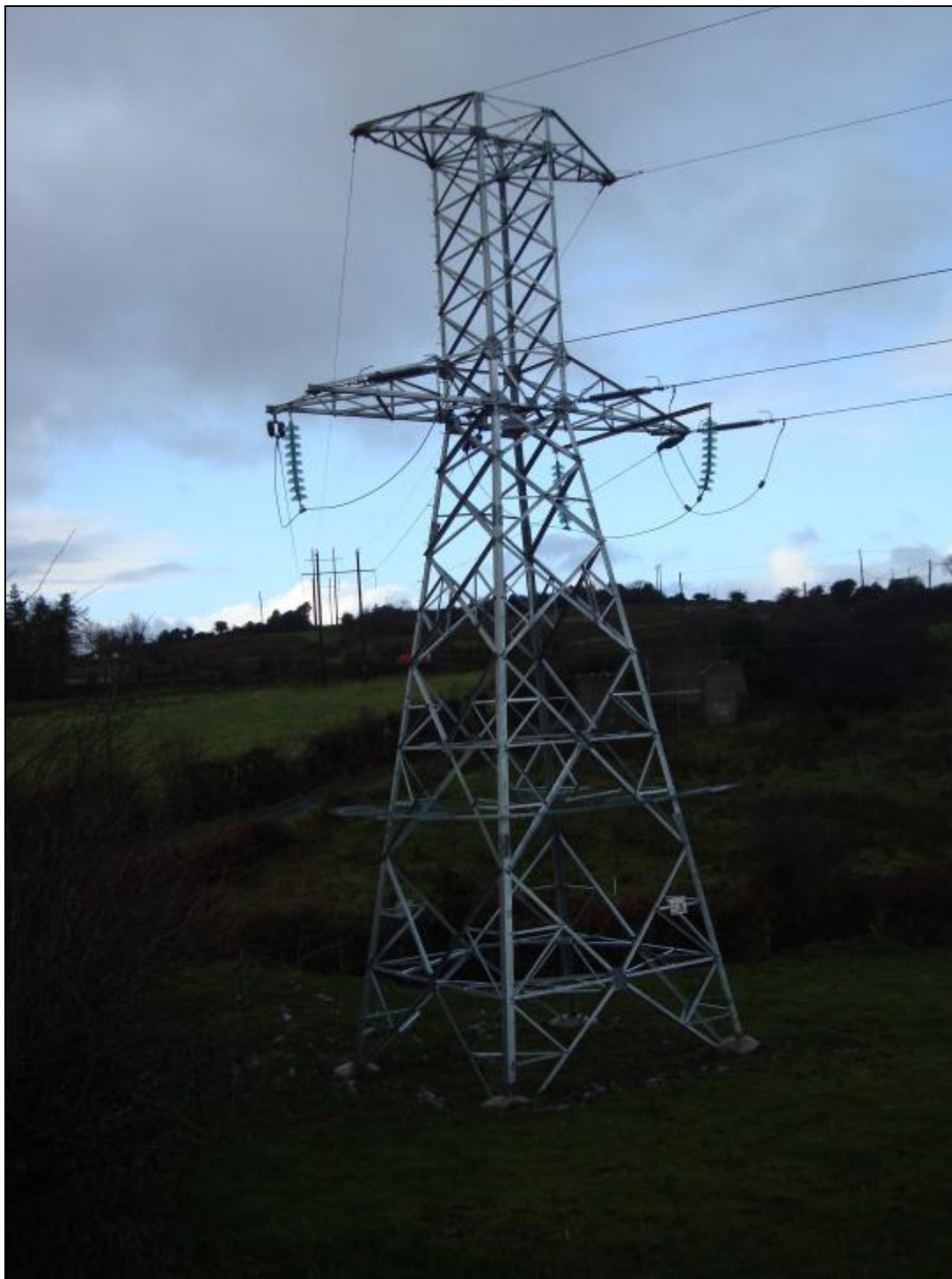
Figure 8.7: Photograph of a 110 kV Earthwire Angle Mast
