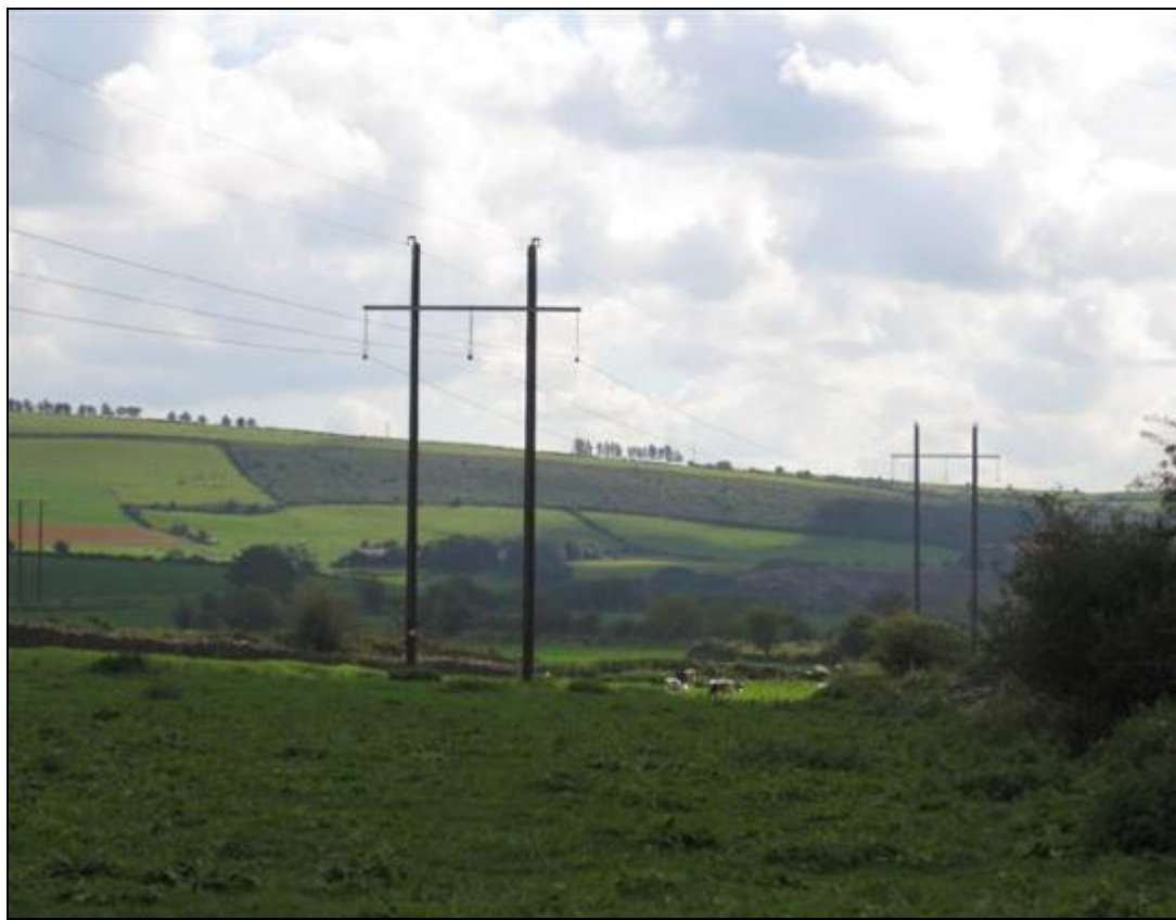
Figure 8.8: Photograph of a 110 kV Earthwire Poleset
