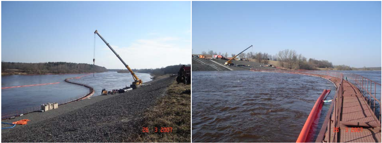
Figure 2.9. Pictures of the stationary barrier to retain oil on the Zapadnaya Dvina River.
