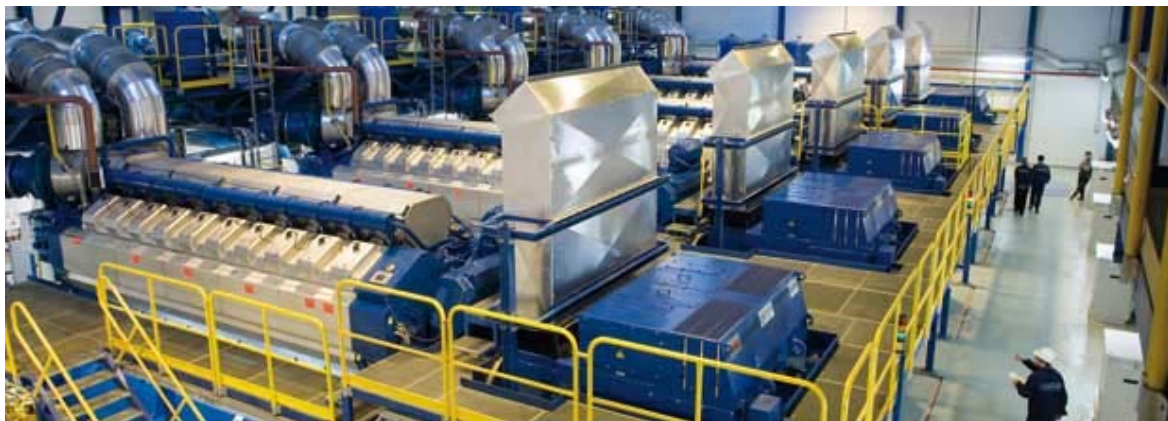
Figure 1: Typical diesel generation plant
