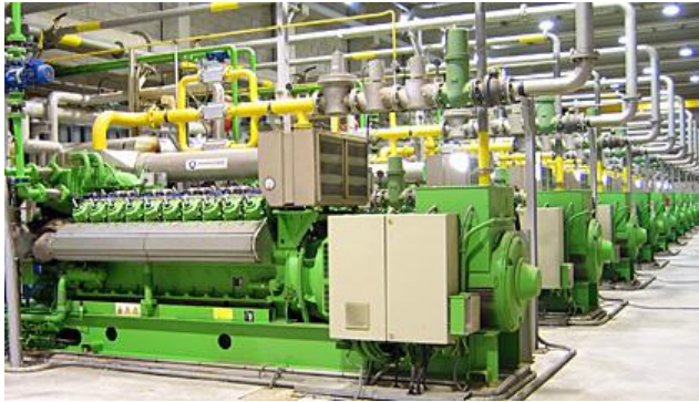
Energy and gas production
