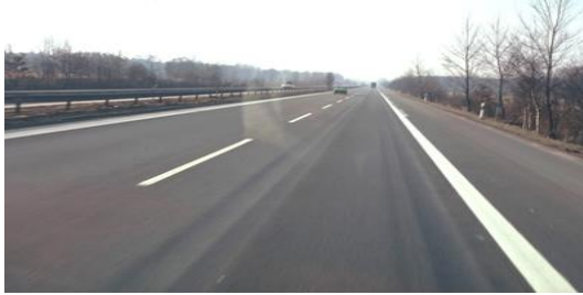
Increase in rutting
