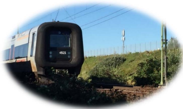
The overhead wire is down
