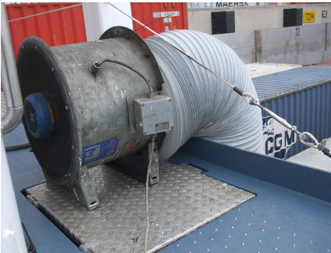
Mobile ventilation system and extraction hose which have been placed on deck above the back of the hold.
