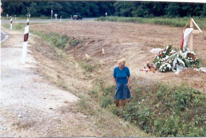
Figure A3. The ditch where the bus landed. Considerable soil deformation can be observed.
