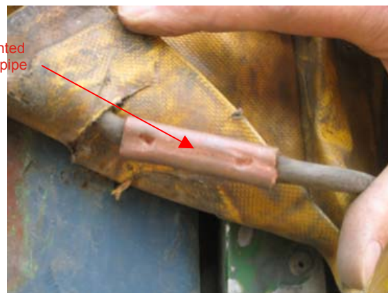
B: TIR-wire repaired with a piece of copper pipe. Note the shiny copper - when was it last replaced?
