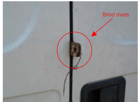
B: Sealing device - rear doors – only fixed with blind rivets.
