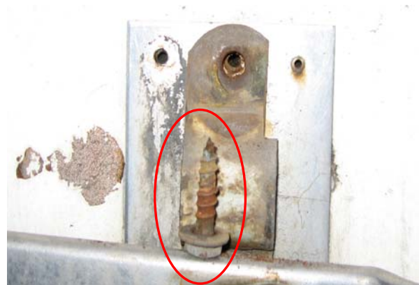
D: The pivoting section secured by a normal Lag bolt meant for wood. The bolt is easily removed and the pivoting section lowered – still attached to the back plate via the string for the Customs seal. The handle is free and can now be operated and the door opened.
