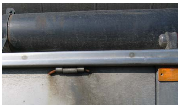
D: Inspect the hinges. The pin for this hinge has been replaced by a piece of rusty iron bar - not secure at all.
