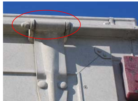
C: Non-secure hinge for the wooden plate. The pin is just a standard bolt with a dome-nut, not welded.
