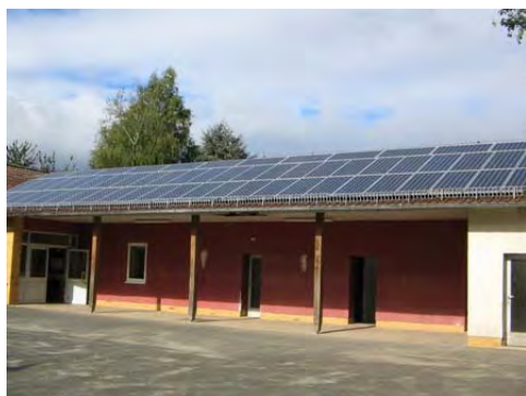
Photovoltaic installation on the roof of the primary school at Fritzlar-Lohne (SEK) with a capacity of 10,8 kWp.
