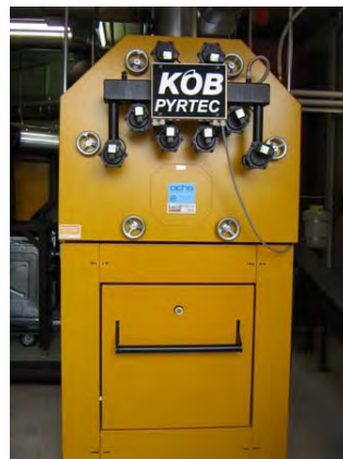
Wood boiler in the secondary school "Gudensberg" with heating capacity of 500 kW
