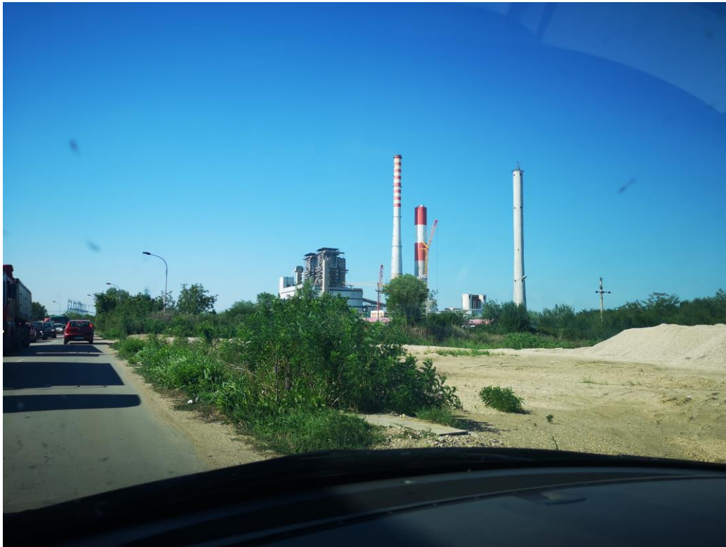
13 August 2019 – the above picture clearly shows the chimney for Kostolac B3 and the cranes that are working on the construction for Kostolac B3.
