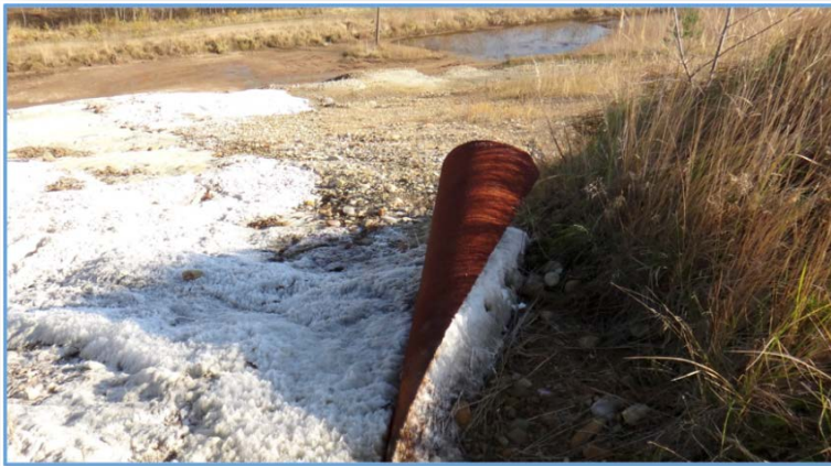
Salt water seepage through the dam
