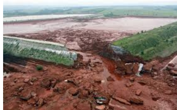
The TMF at Ajkai (Hungary) after the dam failure (2010)
