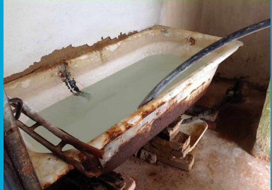
Head works chlorination unit using a bath tub
