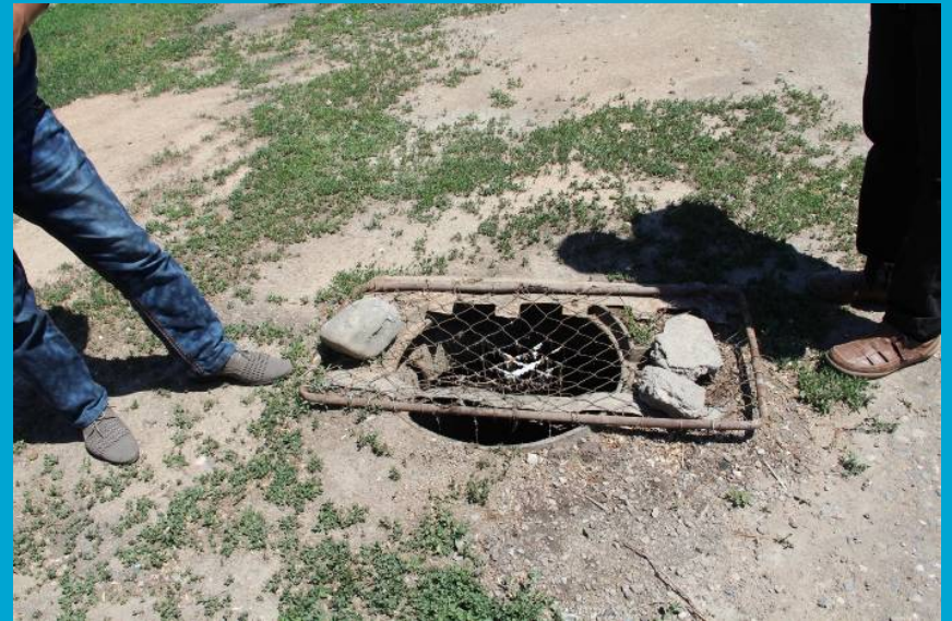
Manhole covers are missing and/or broken
