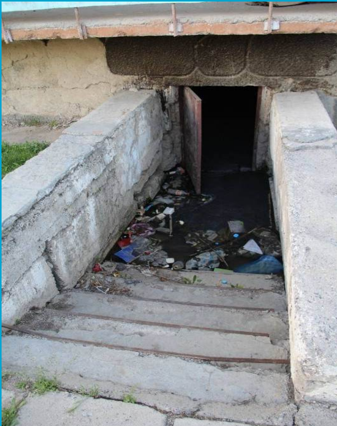
Talas, KR: Sewage from main sewer permanently inundates the basement of a multi-storey building housing 100 people
