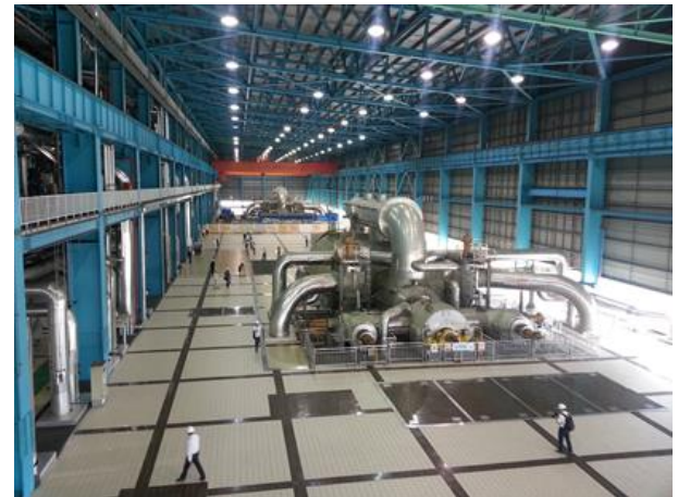
China: Waigaoqiao No3 Power Station, Pudong New Area of Shanghai – 500MW
