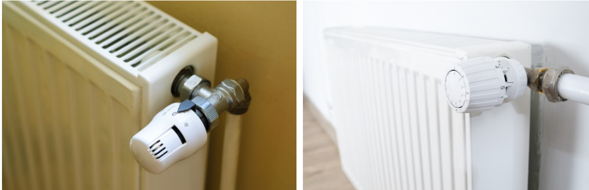
Figure 10. Thermostatic radiator control elements
