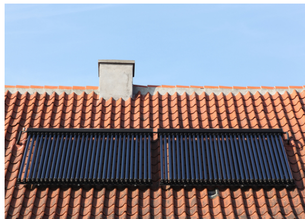
Active solar system with vacuum-tube collectors
