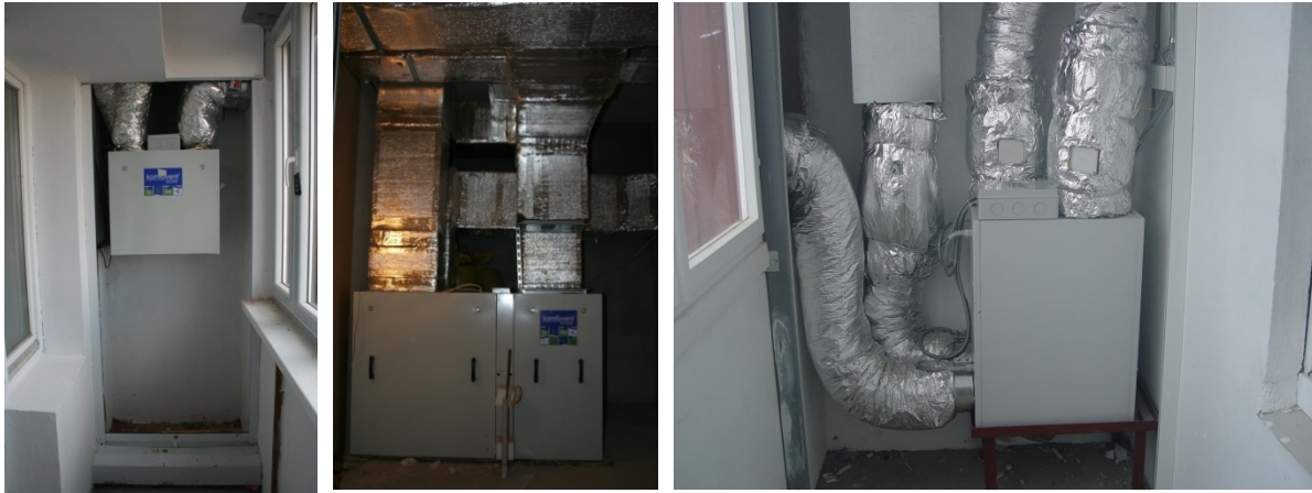
Figure 13. Heat recovery unit for mechanical inlet and outlet ventilation
